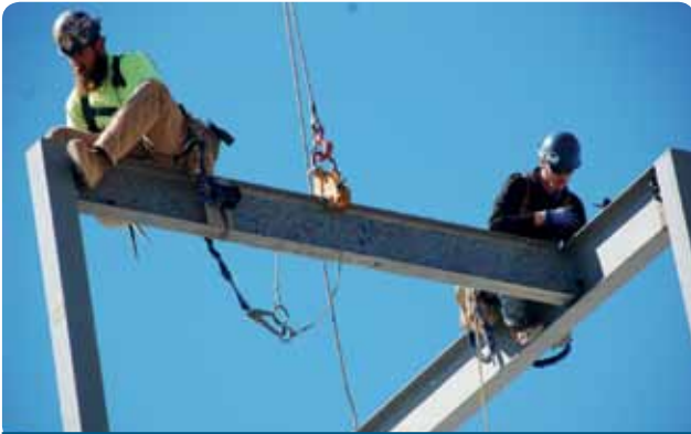
The final beam is installed in the new Wheat Ridge Apartment building.
