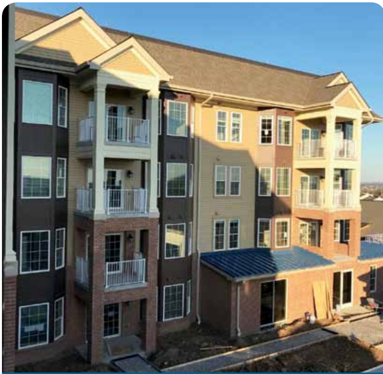
Pictured is a view of the courtyard side of the new Wheat Ridge Apartments. The courtyard will feature a fire pit and bocce court.
